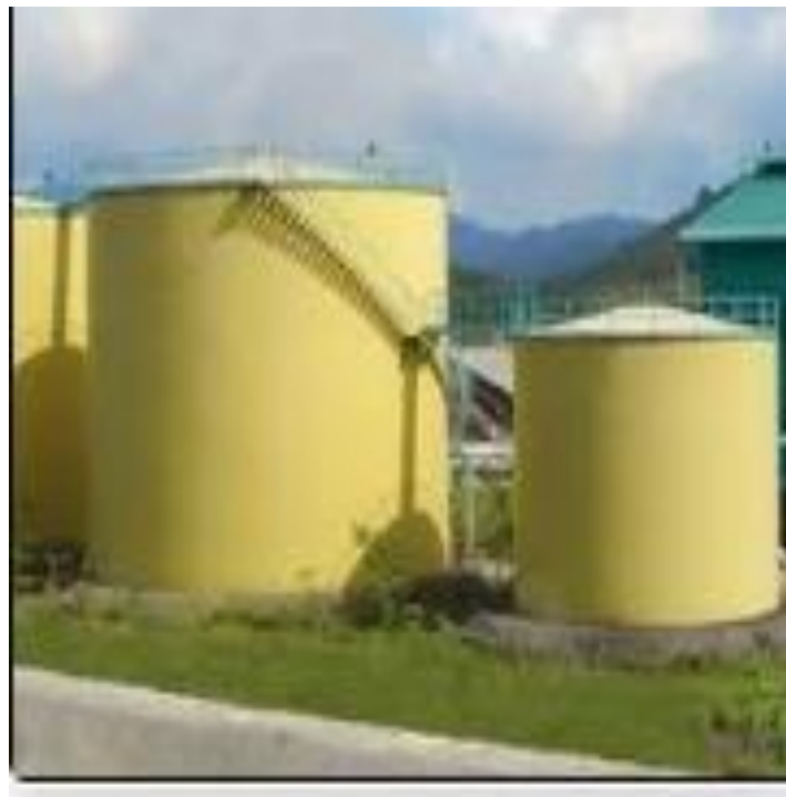
Figure 1. storage tank of crude oil
